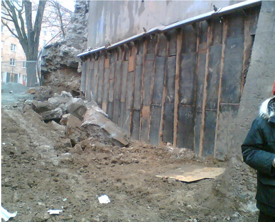
Fig 4. A finalized drilled micro pile wall which, after its role as a temporary structure is completed will support a permanent building.
